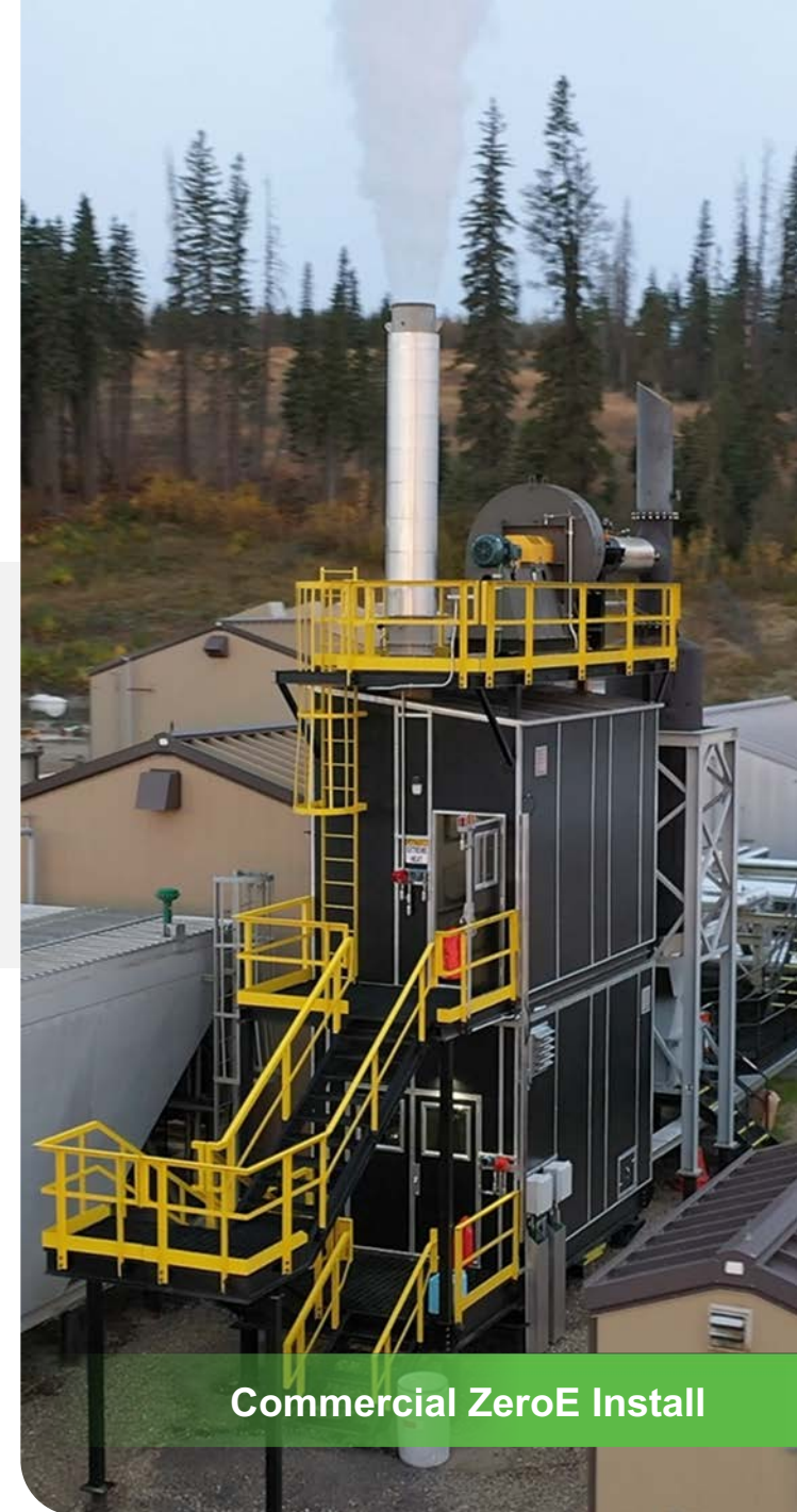
Pilot Demonstration ZeroE Unit
